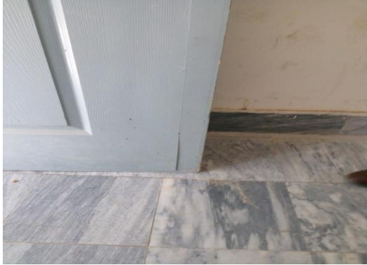
Ply door surface has been disturbed at its erection phase.
