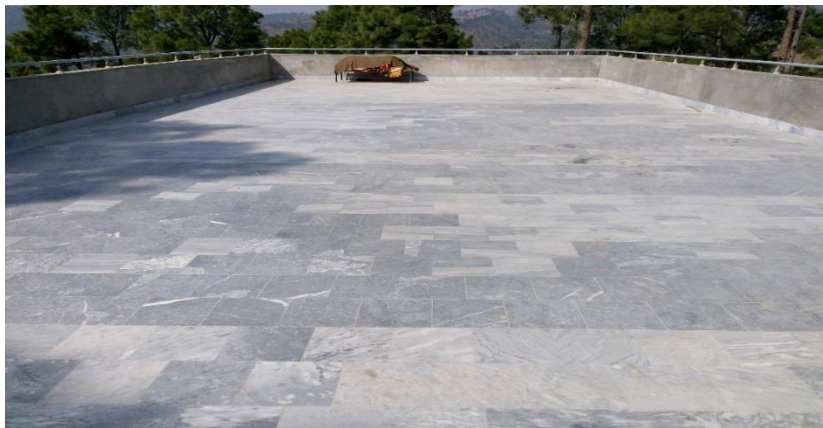
Marble tiles on slab roof of a room has been executed instead insulation. In the BoQ, roof insulation has been proposed.
